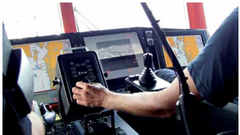
In the Stormbull's cabin two multifunction displays and one dedicated display give all three crewmembers continual access to the Voyager's thermal images. The ergonomic Joystick Control Unit (JCU) is mounted in the middle.
